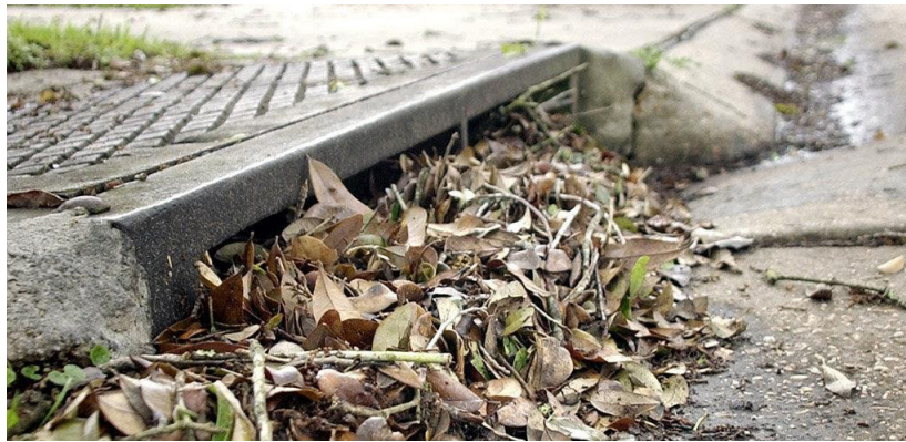
Avoiding this scene means helping to avoid flooding
